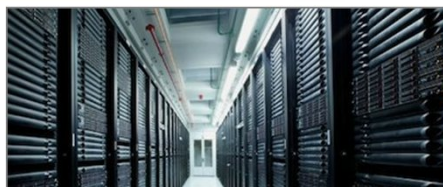
Cloud Data Center
